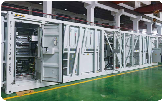
> 45MW/180MWh ESS Project for PV Plant (Spain)
