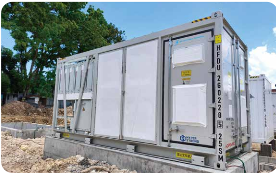
> 92.5MW String ESS Project (Philippines)
