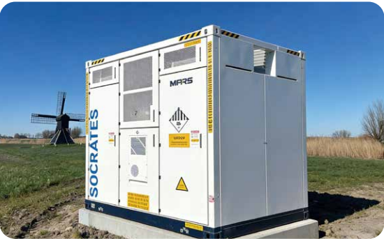
> 4.8MW/9.6MWh ESS Project (Netherlands)
