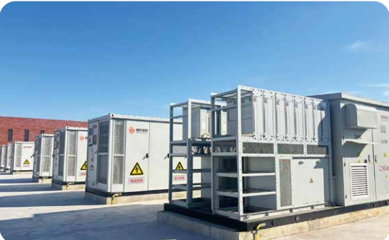
> 25MW/50MWh (Tangshan, Hebei, China)
