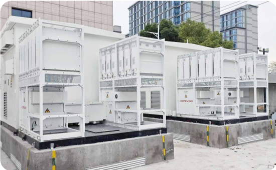
> 5MW/10MWh (Jiaxing, Zhejiang, China)
