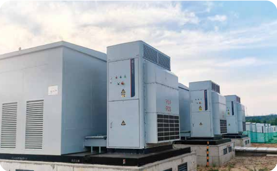
> 307MW/723MWh (Chengde, Hebei, China)
