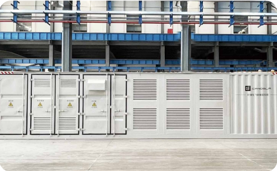
> 1MW flywheel system integration
