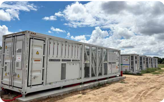
> 12.5MW ESS Project for PV Plant (Spain)
