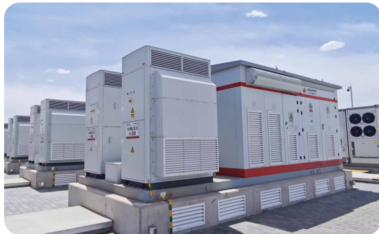
> 160MW/320MWh (Zhongwei, Ningxia, China)
