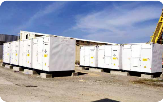
> 5.6MW/11.2MWh ESS Project (Spain)
