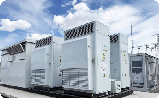
> 200MW/400MW grid-forming (Xilingol, Inner Mongolia, China)
