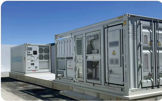
> 2.5MW/5MWh Energy Storage Project (Italy)
