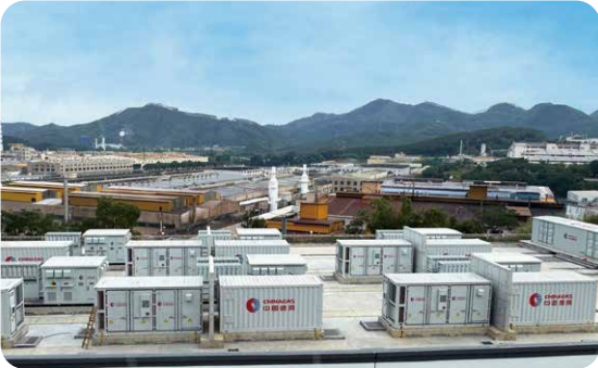
> 25MW/50MWh (Shaoguan, Guangdong, China)
