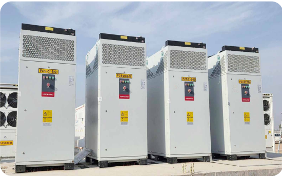
> 360MW ESS Project for PV Plant (India)
