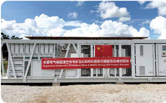
> 4.4MW/8.9MWh Mine On/Off-Grid ESS Project (Zimbabwe)
