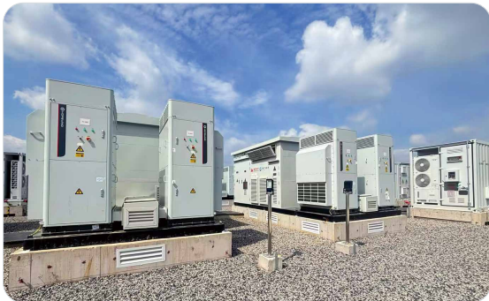
> 100MW/400MWh (Handan, Hebei, China)
