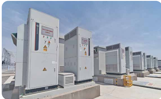
> 100MW/200MWh (Shizuishan, Ningxia, China)
