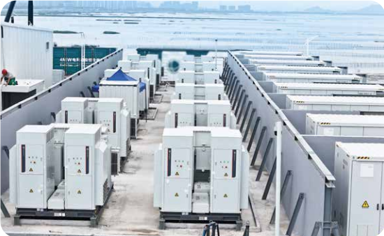
> 52.5MW/105MWh (Yueqing, Zhejiang, China)
