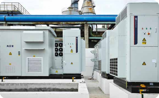
> 50MW/100MWh (Jiangyin, Jiangsu, China)
