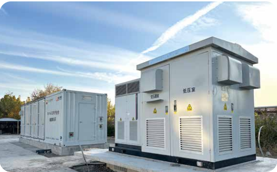
> Dagang oilfield 1MW/1MWh sodium-ion battery (Tianjin, China)
