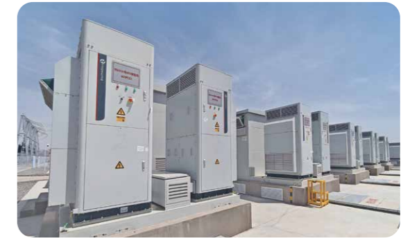
> 100MW/200MWh (Shizuishan, Ningxia, China)
