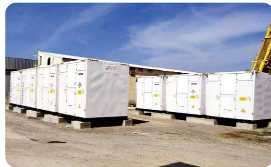
> 5.6MW/11.2MWh ESS Project (Spain)
