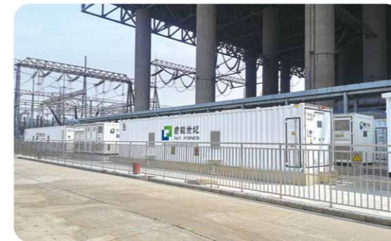
> 15MW/7.5MWh thermal power plant ESS (Shanxi, China)
