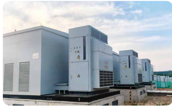
> 307MW/723MWh (Chengde, Hebei, China)
