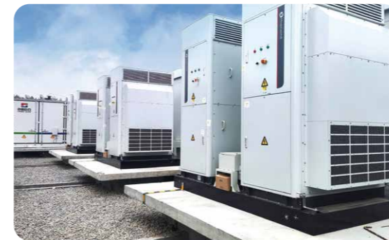
> 23MW/46MWh (Lianshui, Jiangsu, China)
