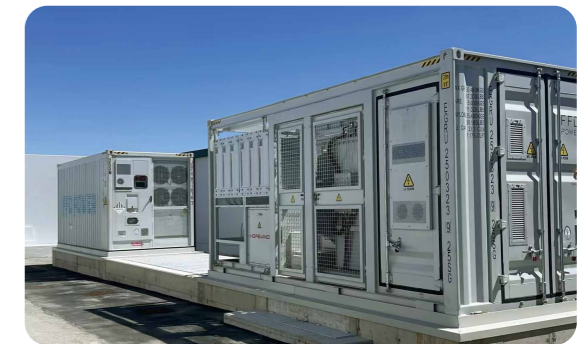
> 2.5MW/5MWh Energy Storage Project (Italy)
