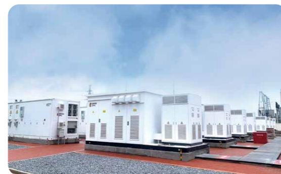
> 100MW/200MWh (Zhucheng, Shandong, China)
