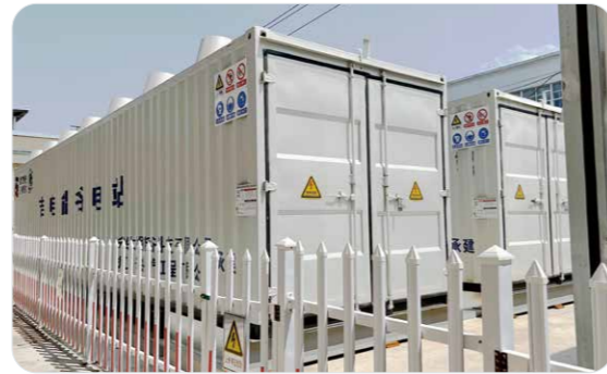
> 3MW/31MWh lead-carbon battery project (Changxing, Zhejiang, China)
