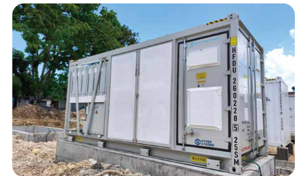
> 92.5MW String ESS Project (Philippines)
