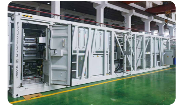
> 45MW/180MWh ESS Project for PV Plant (Spain)
