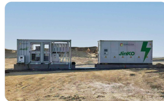
> 1.25MW/2.5MWh C&I ESS Project for PV Plant (Egypt)
