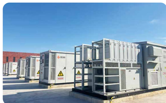
> 25MW/50MWh (Tangshan, Hebei, China)
