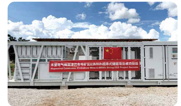
> 4.4MW/8.9MWh Mine On/Off-Grid ESS Project (Zimbabwe)
