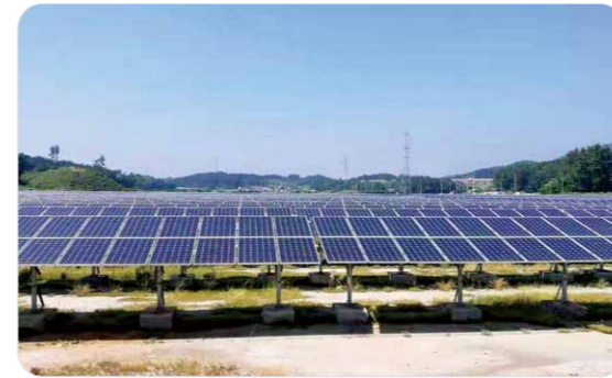
> 12MW/36MWh ESS Project for PV Plant (South Korea)
