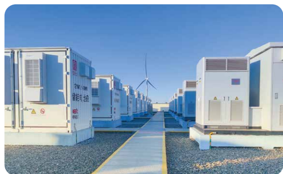
> 120MW/240MWh (Alashan, Inner Mongolia, China)
