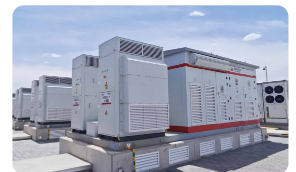
> 160MW/320MWh (Zhongwei, Ningxia, China)
