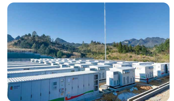
> 100MW/200MWh (Qiannan, Guizhou, China)
