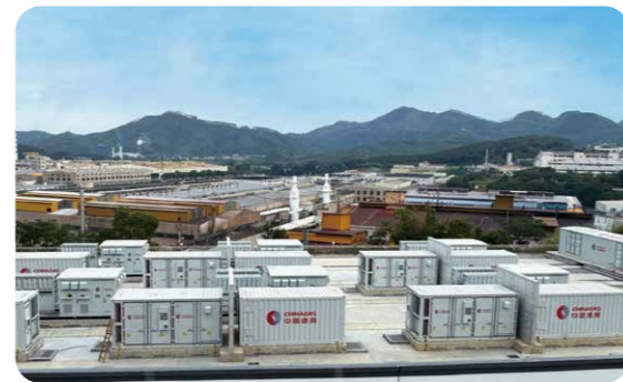
> 25MW/50MWh (Shaoguan, Guangdong, China)
