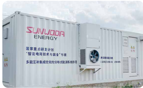
> 3MW/6MWh (Huizhou, Guangdong, China)
