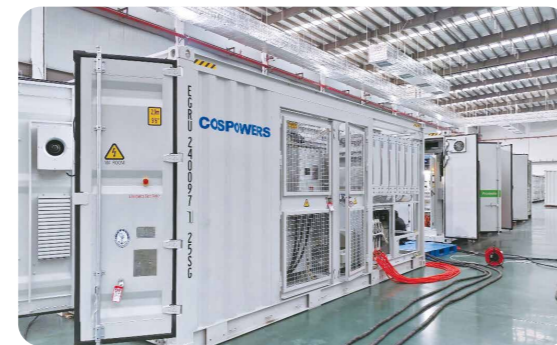
> 2.5MW/5MWh PCS Turnkey Station (Latvia)
