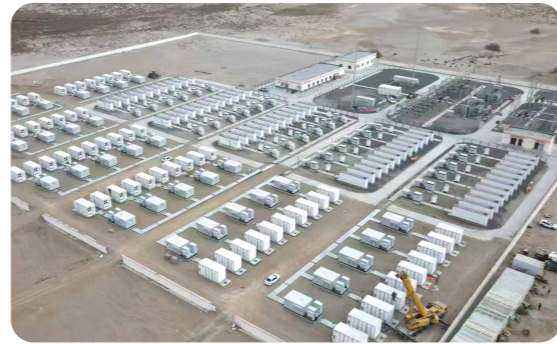
> 180MW/360MWh (Jiuquan, Gansu, China)
