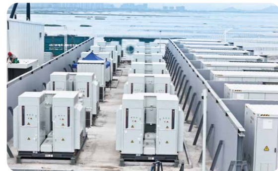
> 52.5MW/105MWh (Yueqing, Zhejiang, China)
