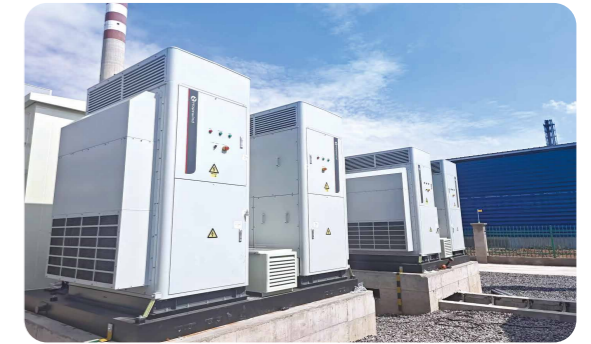
> 25MW/50MWh (Fuyang, Anhui, China)
