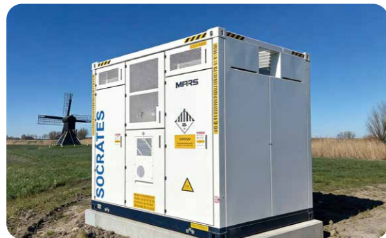
> 4.8MW/9.6MWh ESS Project (Netherlands)
