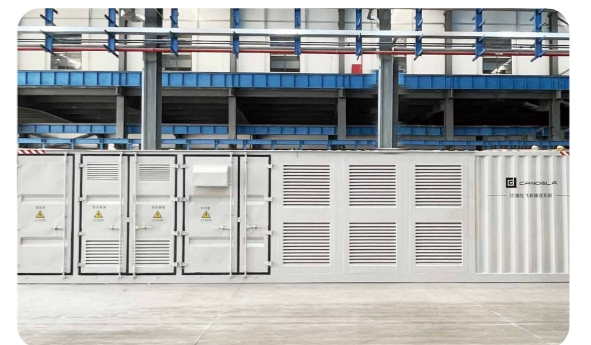
> 1MW flywheel system integration
