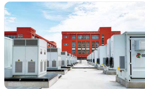
> 100MW/200MWh (Jining, Shandong, China)
