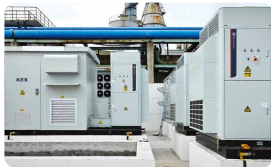
> 50MW/100MWh (Jiangyin, Jiangsu, China)
