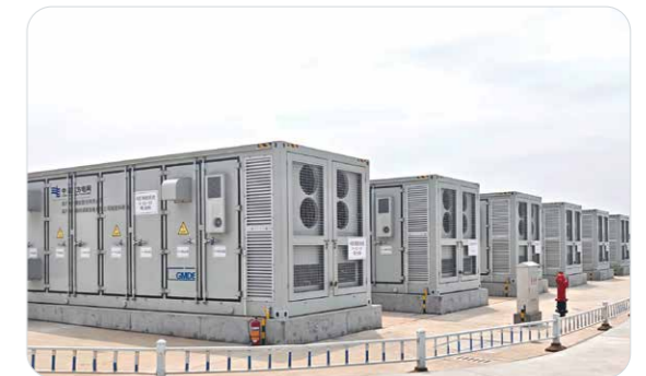
> 20MW/40MWh grid-forming (Wenshan, Yunnan, China)
