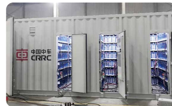
> Supercapacitor energy storage
