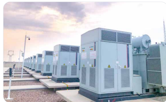
> 150MW/300MWh (Yinchuan, Ningxia, China)
