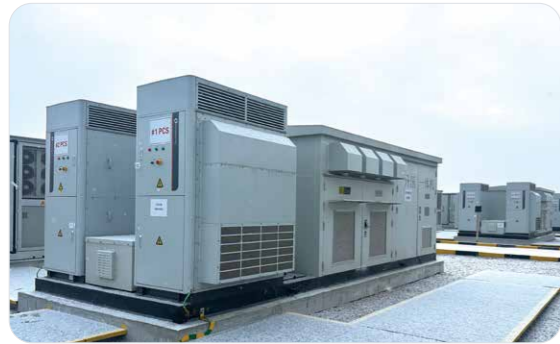
> 250MW/1000MWh (Aral, Xinjiang, China)
