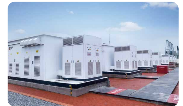
> 100MW/200MWh (Dongming, Shandong, China)
