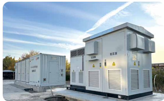
> Dagang oilfield 1MW/1MWh sodium-ion battery (Tianjin, China)
