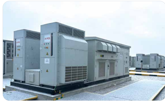
> 250MW/1000MWh (Aral, Xinjiang, China)
