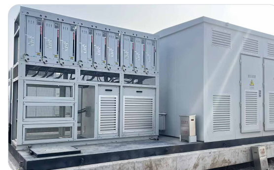
> 100MW/200MWh (Jiuquan, Gansu, China)
