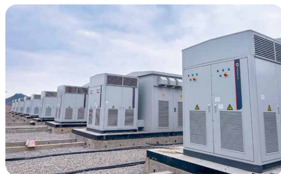
> 100MW/200MWh (Anshun, Guizhou, China)
