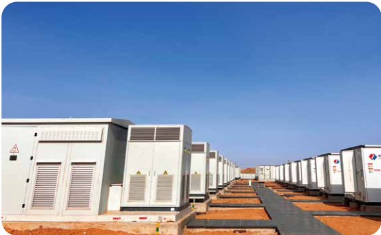
> 50MW/100MWh (Wuzhong, Ningxia, China)
