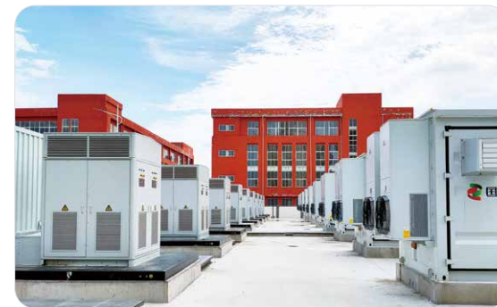
> 100MW/200MWh (Jining, Shandong, China)
