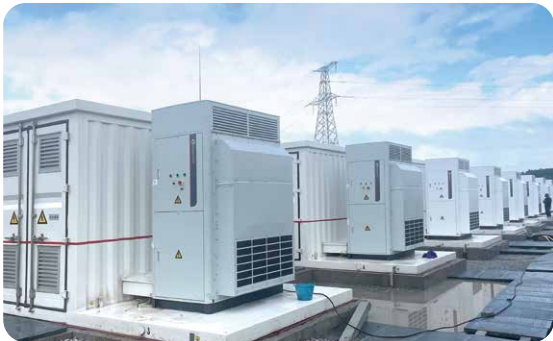
> 25MW/50MWh (Ledong, Hainan, China)
