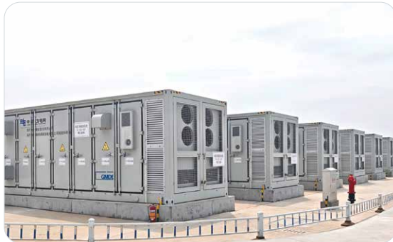
> 20MW/40MWh grid-forming (Wenshan, Yunnan, China)
