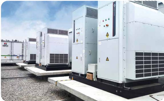
> 23MW/46MWh (Lianshui, Jiangsu, China)
