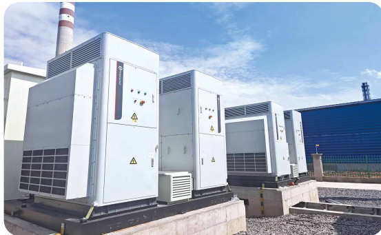
> 25MW/50MWh (Fuyang, Anhui, China)
