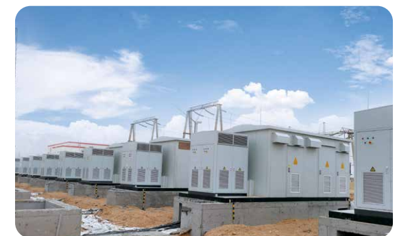
> 60MW/120MWh (Alxa, Inner Mongolia, China)
