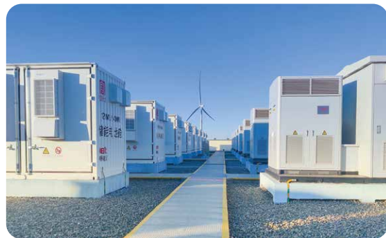
> 120MW/240MWh (Alashan, Inner Mongolia, China)
