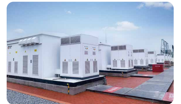
> 100MW/200MWh (Dongming, Shandong, China)
