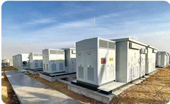
> 50MW/100MWh (Hulunbuir, Inner Mongolia, China)
