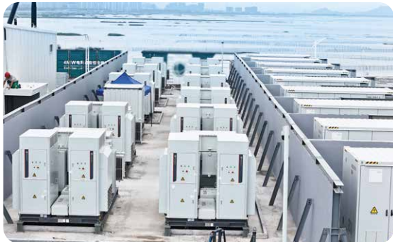
> 52.5MW/105MWh (Yueqing, Zhejiang, China)
