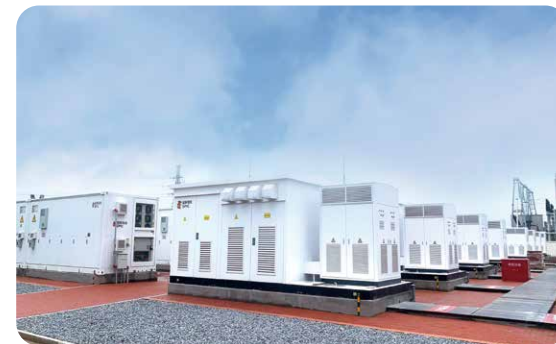
> 100MW/200MWh (Zhucheng, Shandong, China)
