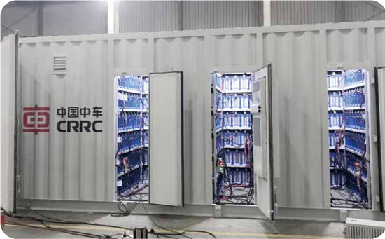
> Supercapacitor energy storage
