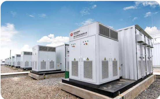
> 57.5MW/115MWh (Xiantao, Hubei, China)
