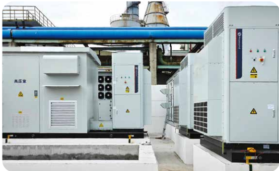
> 50MW/100MWh (Jiangyin, Jiangsu, China)
