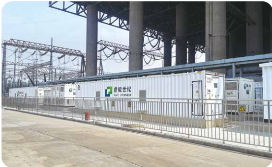
> 15MW/7.5MWh thermal power plant ESS (Shanxi, China)
