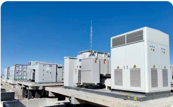
> 40MW/80MWh (Jiuquan, Gansu, China)
