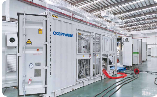
> 2.5MW/5MWh PCS Turnkey Station (Latvia)
