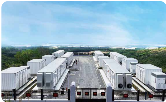
> 25MW/50MWh (Ledong, Hainan, China)
