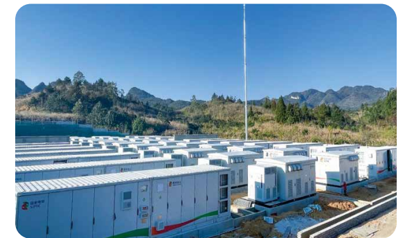
> 100MW/200MWh (Qiannan, Guizhou, China)
