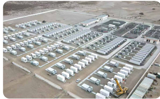
> 180MW/360MWh (Jiuquan, Gansu, China)
