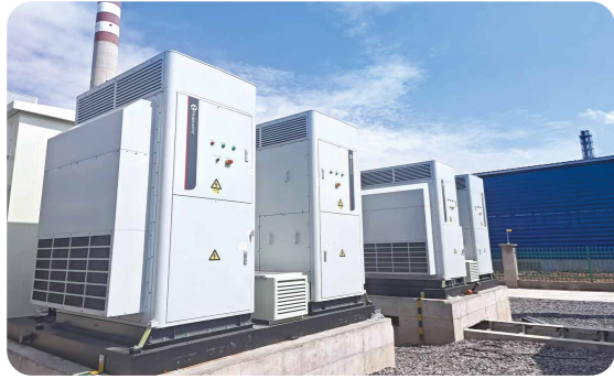
> 25MW/50MWh C&I energy storage project in Fuyang, Anhui province
