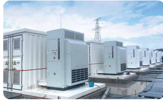
> 25MW/50MWh generator-side energy storage project in Wanning, Hainan province
