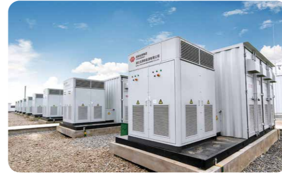
> 57.5MW/115MWh Generator-side energy storage project in Xiantiao city, Hubei province
