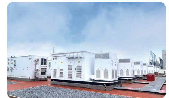
> 100MW/200MWh energy storage project in Zhucheng, Shandong province
