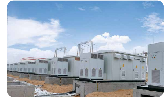
> 60MW/120MWh Generator-side energy storage project in Alxa League, Inner Mongolia
