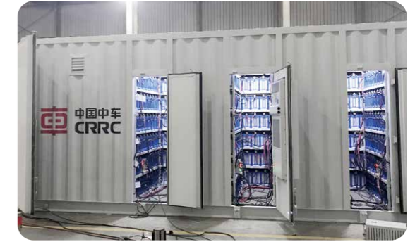
> Supercapacitor Energy Storage
