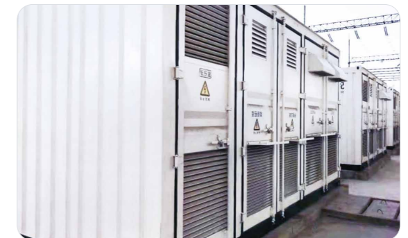
> Energy storage EMS project of a metal factory in Jiangyin City, Jiangsu Province
