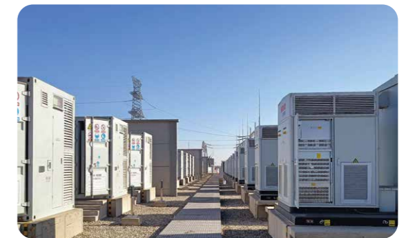
> 154MW/308MWh energy storage project in Jiayuguan, Gansu province
