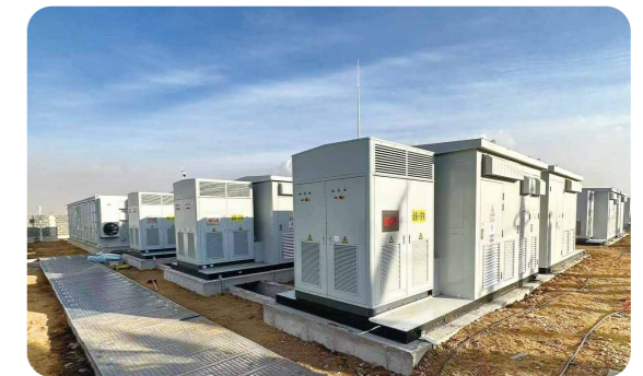
> 50MW/100MWh Generator-side energy storage project in Hulun Buir city, Inner Mongolia
