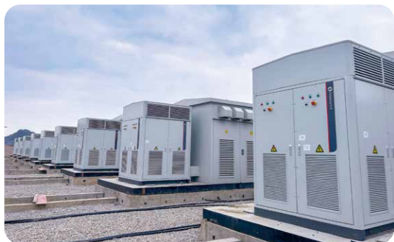
> 100MW/200MWh energy storage project in Anshun, Guizhou province
