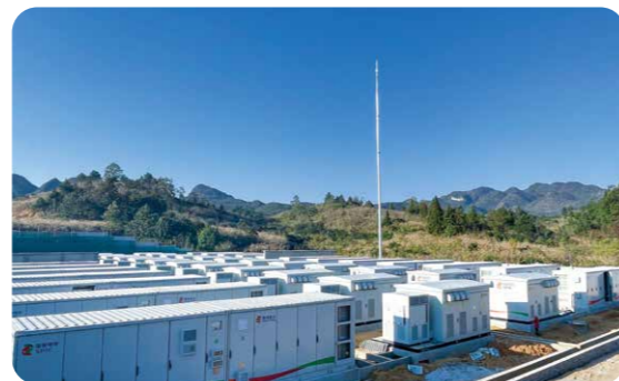
> 100MW/200MWh energy storage project in Luodian, Guizhou province
