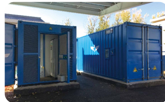
> Micro-grid EMS project in Fangshan District, Beijing
