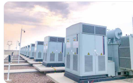
> 150MW/300MWh energy storage project in Yinchuan, Ningxia
