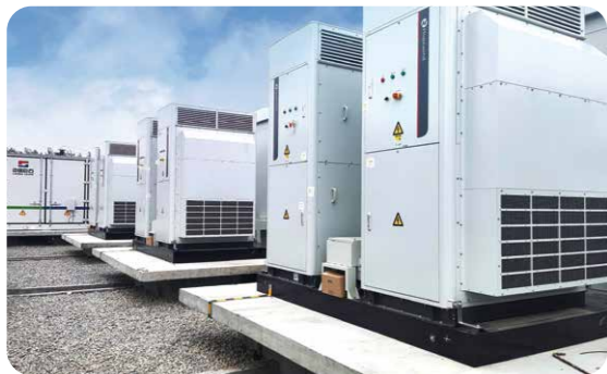
> 23MW/46MWh generator-side energy storage project in Lianshui, Jiangsu province
