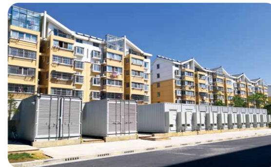
> User-side Energy Storage + UPS Project
