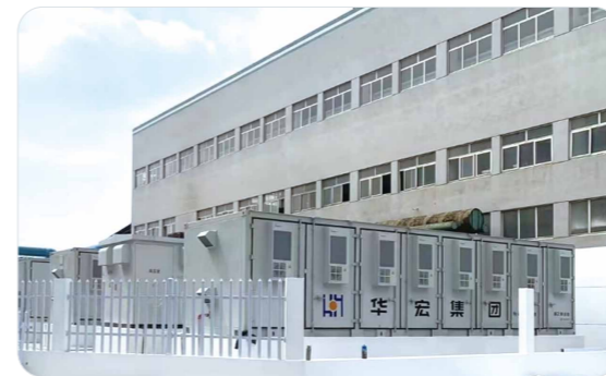
> Energy storage EMS project in Jiangyin City, Jiangsu Province
