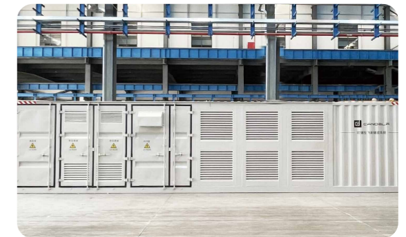
> 1MW Flywheel System Integration
