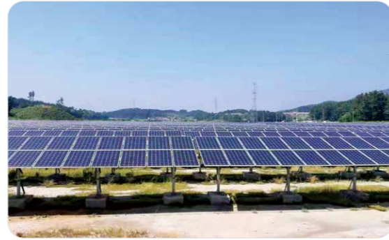
> South Korea 12MW/36MWh Photovoltaic Energy Storage Project
