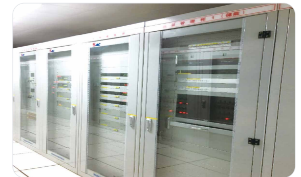
> Wind power distribution and storage EMS project in Luohe City, Henan Province
