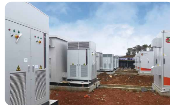
> 100MW/200MWh energy storage project in Weng'an, Guizhou province
